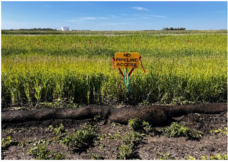
Date: 6/10/2024 Location: Sta. No. 268+30. Notes: Installed No Pipeline Access sign at intersection of construction right-of-way and 165 th Avenue SE in background.
