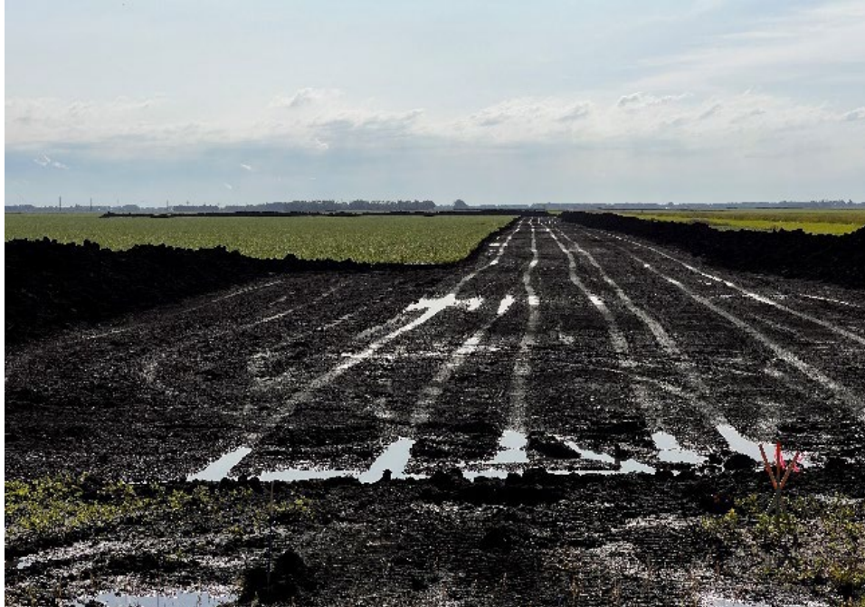
Date: 7/15/2024 Location: Sta. No. 1405+00 Notes: No construction occurred on the construction right-of-way due to a recent rain event.
