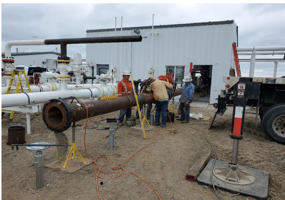
Date: 8/29/2024 Location: Mapleton Compressor Station. Notes: Welding aboveground piping to transfer station.
