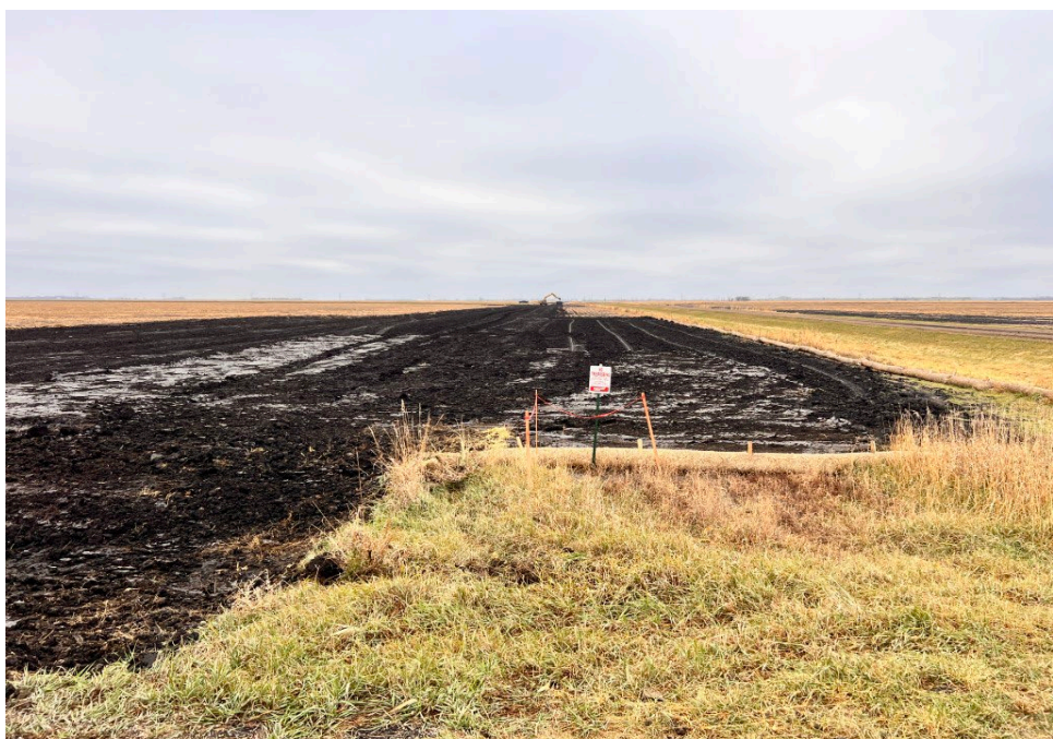
Date: 11/02/2024 Location: Sta. No. 2331 +00 Notes: Looking south across construction right-of-way and additional temporary workspace for Bore 55.
