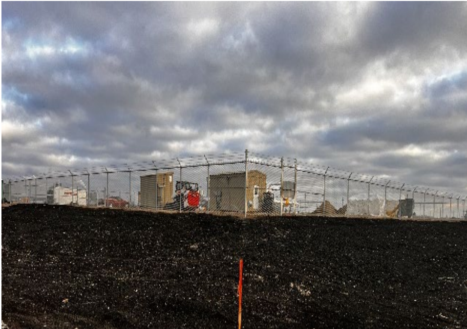
Date: 11/14/2024 Location: Valve Site 7 and MDU-Wahpeton Border Station. Notes: Completed security fence.
