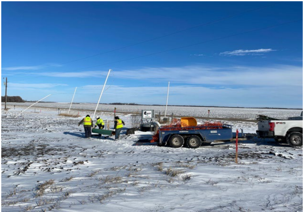
Date: 11/25/2024 Location: Sta. No.2138+00 Notes: Removal of construction debris along the construction right-of-way.
