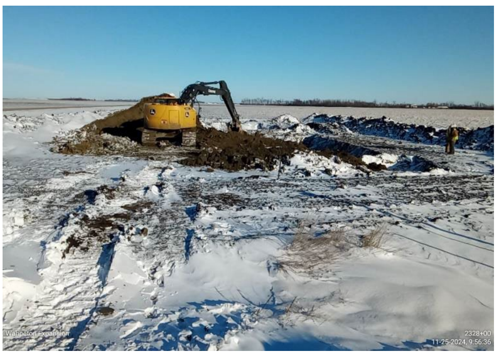
Date: 11/25/2024 Location: Sta. No. 2328+00 Notes: Backfilling after the inspection of an anomaly found in the pipeline.
