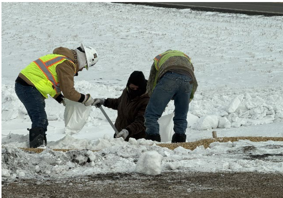
Date: 1/15/2025 Location: MDU- Wahpeton Border Station. Notes: Maintenance of erosion control devices.
