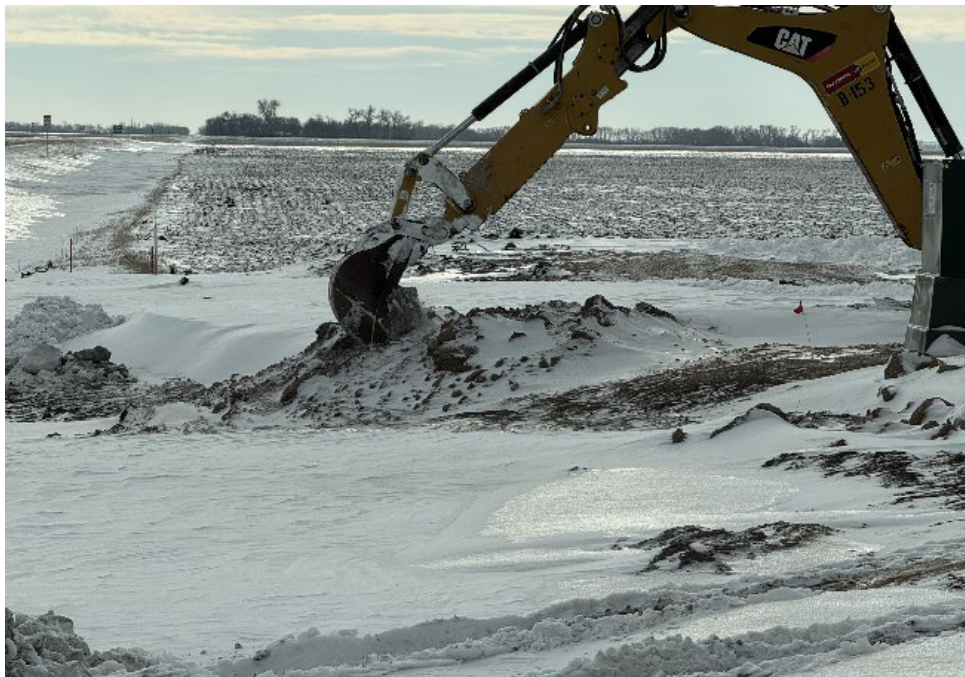
Date: 1/15/2025 Location: MDU- Wahpeton Border Station. Notes: Cleanup of excess construction material left after the local distribution company (MDU) installed their equipment near the border station.
